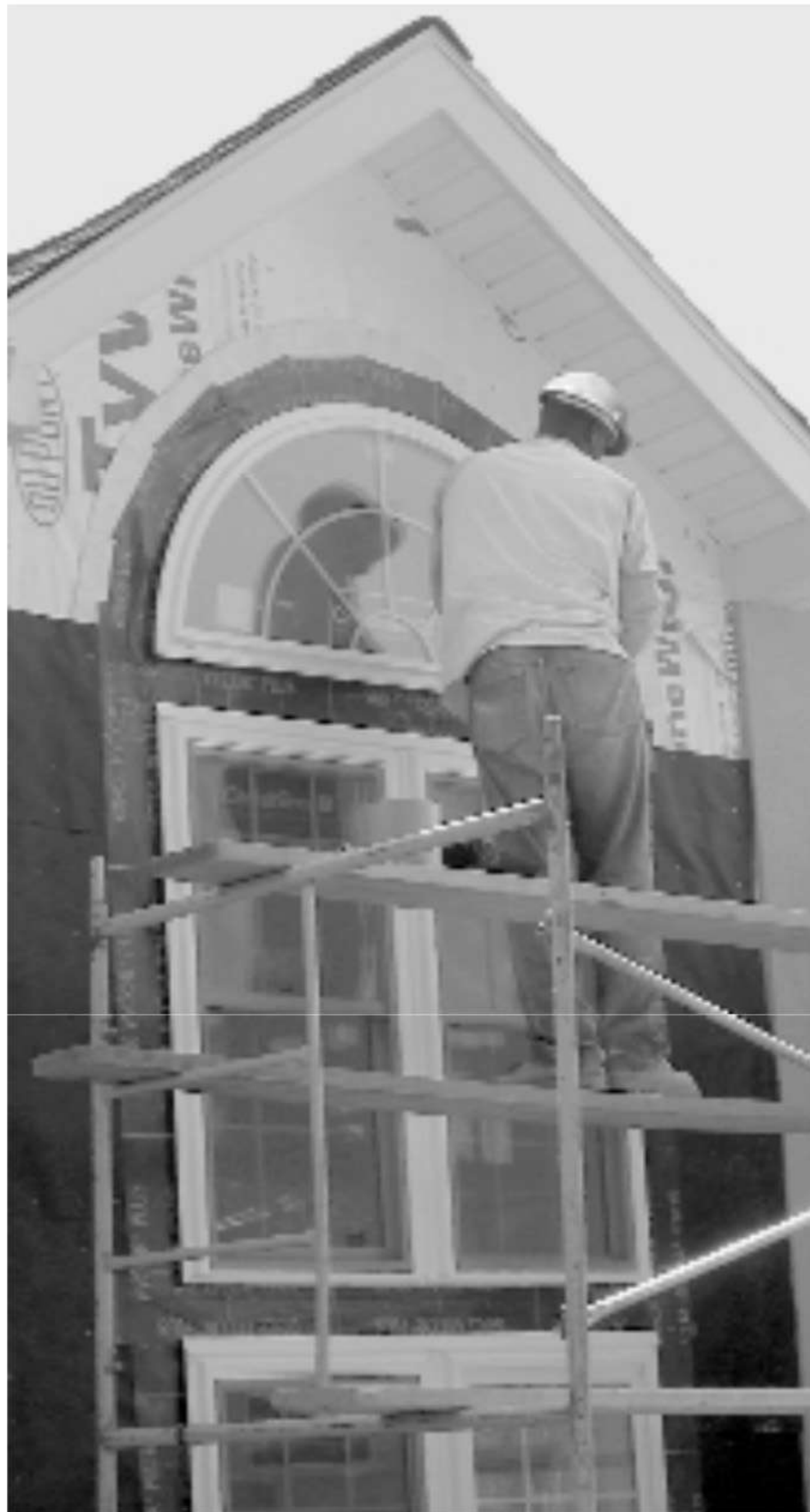
Fig. 1 Cover the area with two layers of weather barrier. Adhere rubber flashing around all openings.
