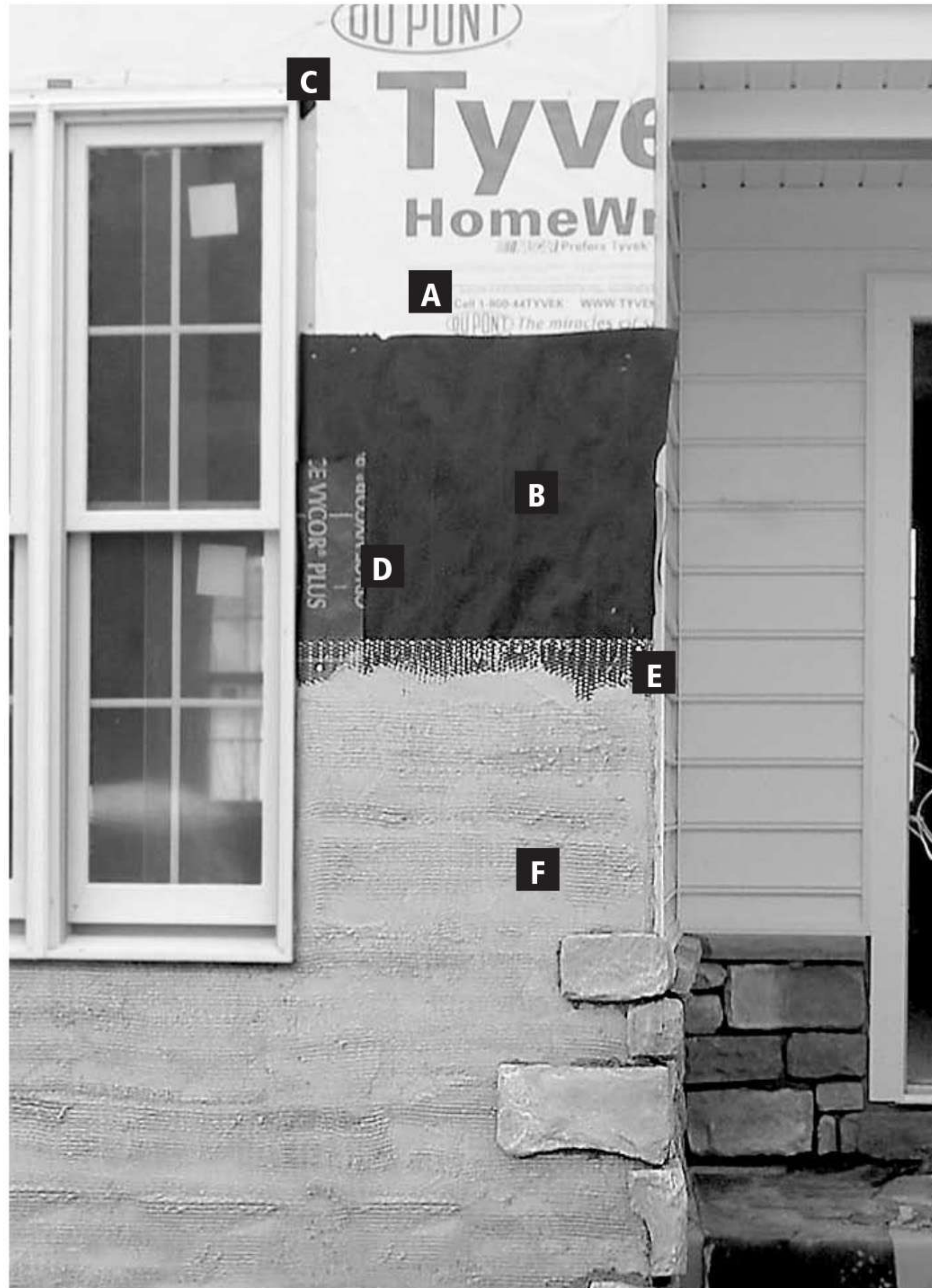
Fig. 5 When preparation is complete, your surface should include: A. a layer of weather barrier (installed by the builder before windows and doors), B. a second layer of weather barrier, C. metal flashing on windows and doors (installed by builder), D. rubber flashing around all openings, E. galvanized metal self-furring lath, and F. a 1/2" scratch coat.
